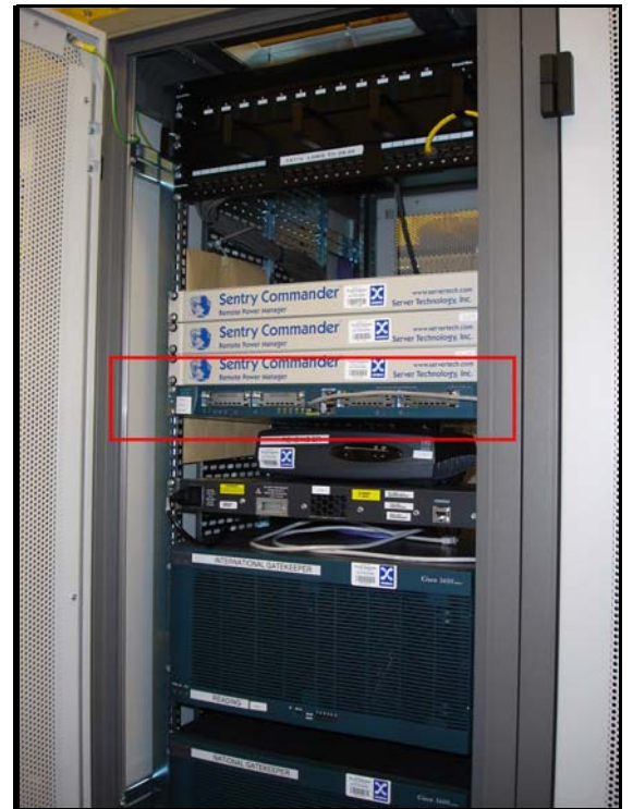
UKERNA Network Monitoring Device installed at Co-location facility
