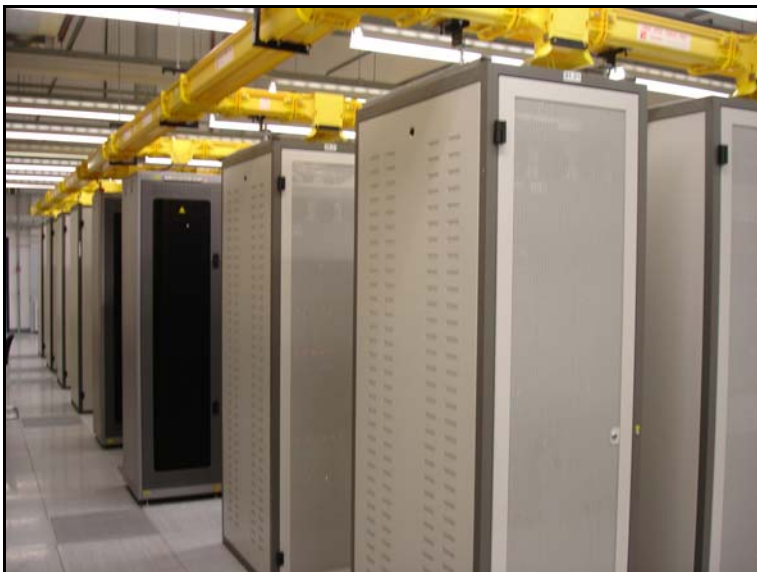
JANET Co-location Facility
